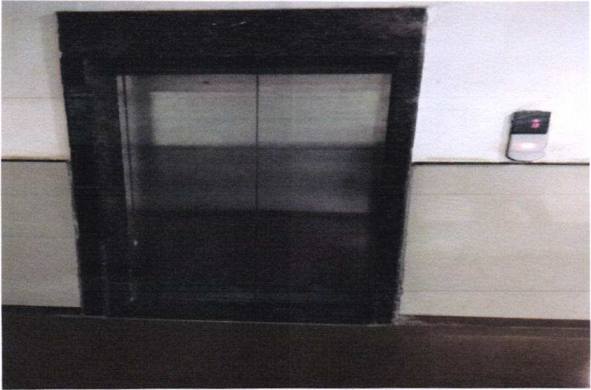
Lift facility for Divyangjan at Common Conference Hall Building
